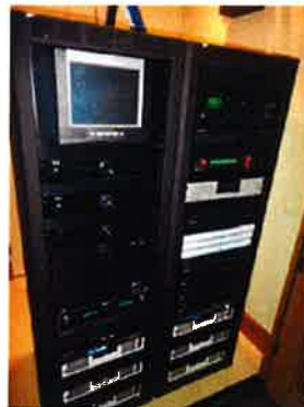
Universal Systems' Austin project incorporates Middle Atlantic Products' gangable WRK Series wide body equipment racks.
